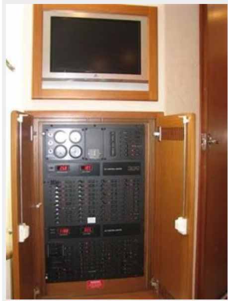
Salon TV & Breaker Panel
