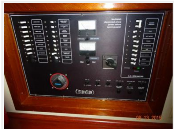
31' Camano electrical panel
