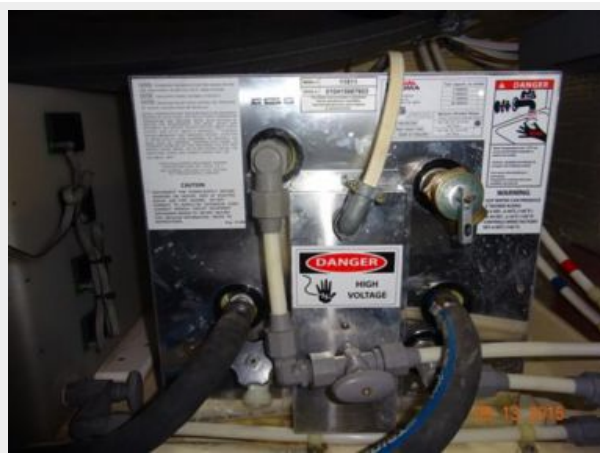
31' Camano water heater
