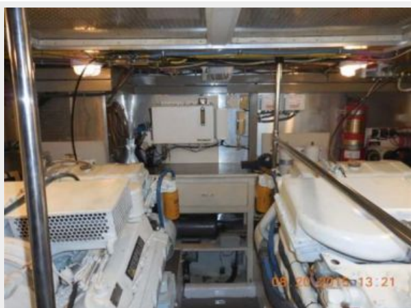
Engine room Forward
