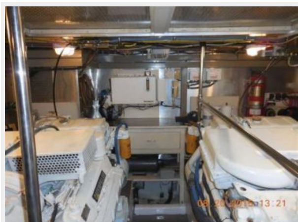
Engine room Forward
