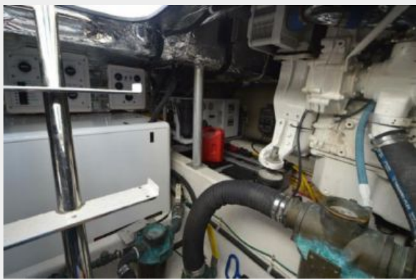
Engine Room and Generator
