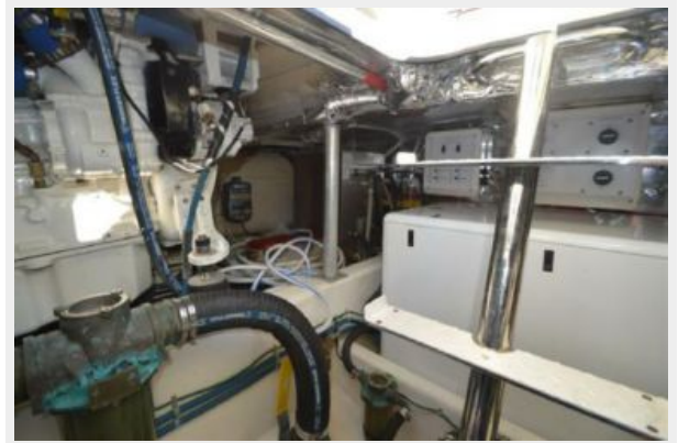
Engine Room and Generator
