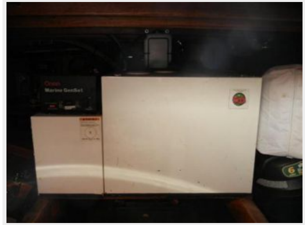
Onan 9.5kw Genset - 1238 hrs.
