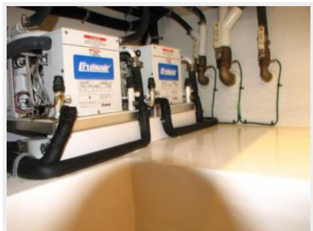
Engine & Mechanical Equipment 4 - AC Units
