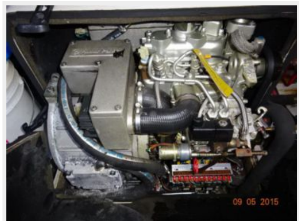
54' Ocean Alexander generator2
