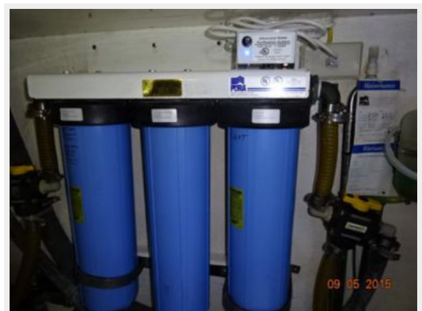
54' Ocean Alexander fresh water system filtration
