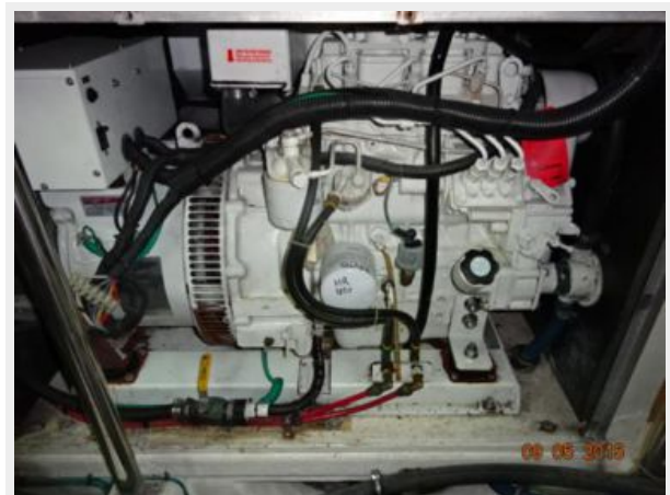
54' Ocean Alexander generator1
