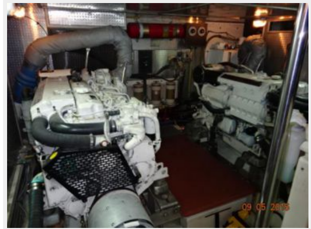
54' Ocean Alexander engine room aft
