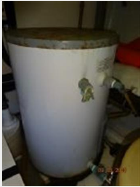
54' Ocean Alexander water heater
