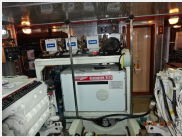
54' Ocean Alexander engine room forward
