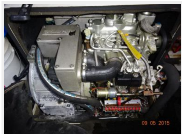
54' Ocean Alexander generator2
