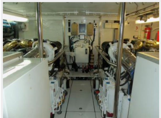
Engine Room Looking Forward
