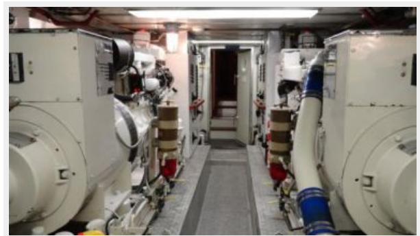
Engine Room Looking Fwd.
