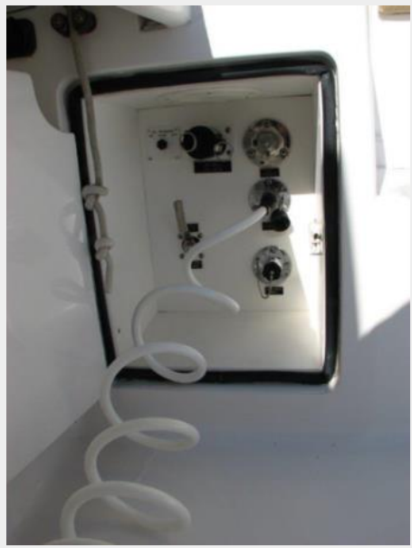
Deck 8 - Port Dockside Box
