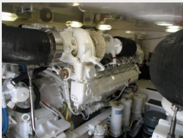
Engine & Mechanical Equipment 1 - Port Engine
