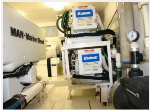
Engine & Mechanical Equipment 4 - Engine Room
