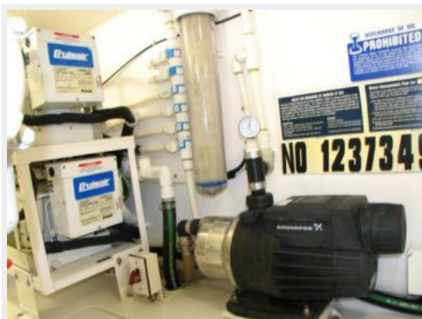
Engine & Mechanical Equipment 5 - Engine Room
