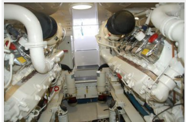
Engine room aft
