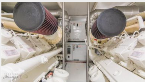
Engine Room Gens
