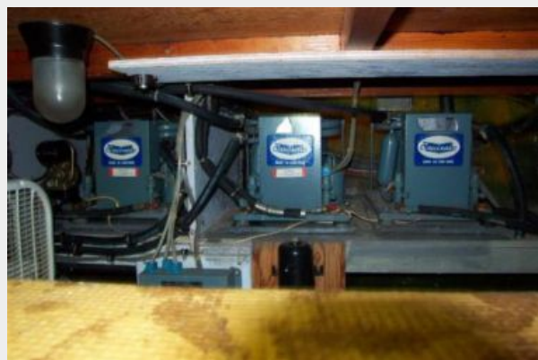
New A/C compressors
