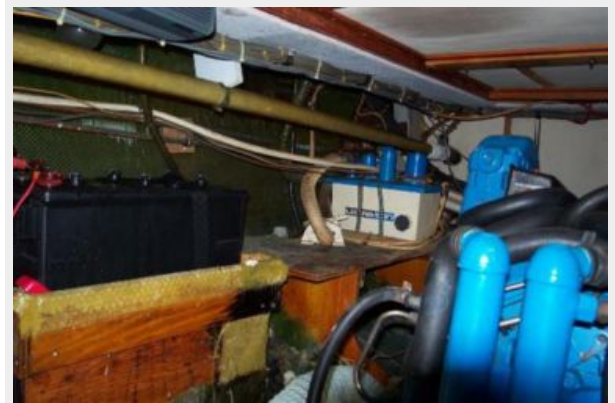
Engine Room-outboard, starboard
