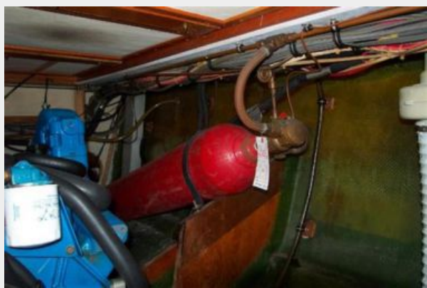
Engine Room-outboard, port
