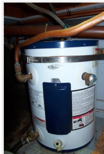
New Hot Water Heater
