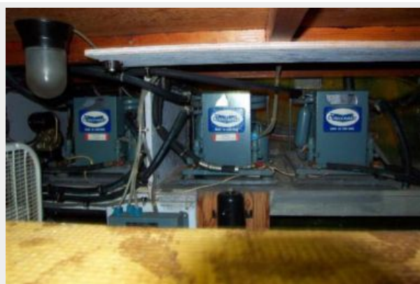
New A/C compressors
