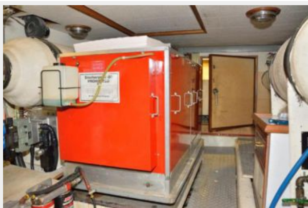
Engine Room Aft - Generator
