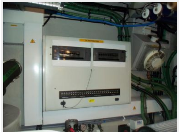
Engine Room Panel
