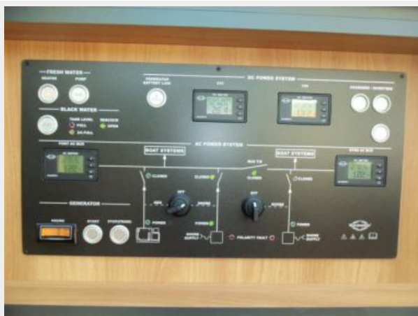
Companionway Electrical Panel
