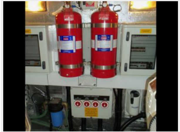
Engine Room Aft
