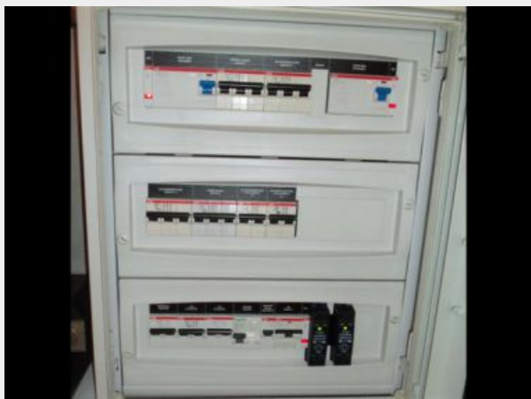
Engine Room Panel
