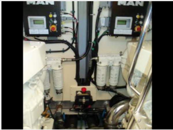
Engine Room Forward
