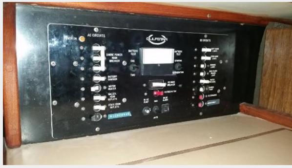
AC/DC Control Panel
