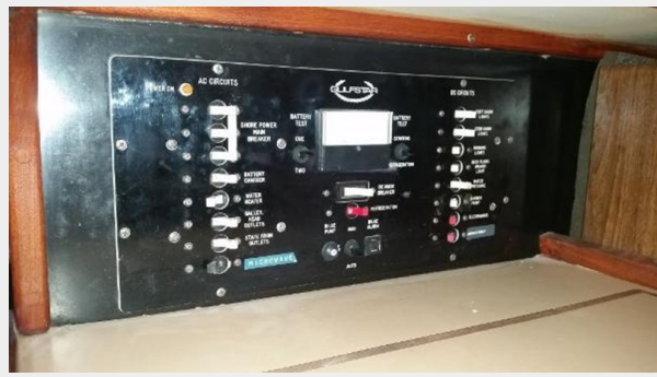
AC/DC Control Panel
