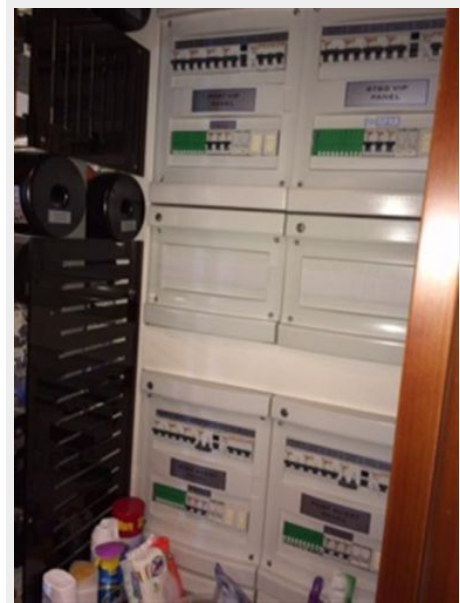
Lower Foyer electrical Panel
