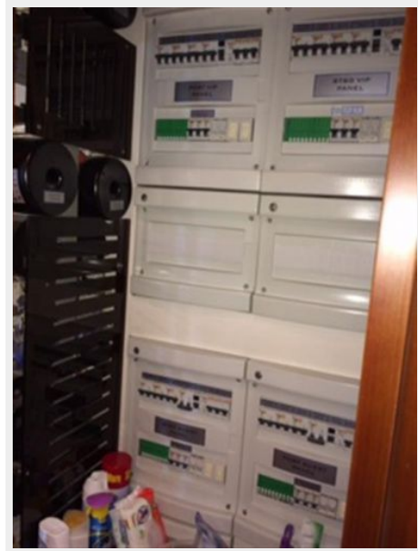
Lower Foyer electrical Panel
