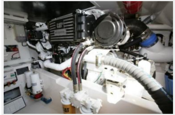
Starboard Main Engine
