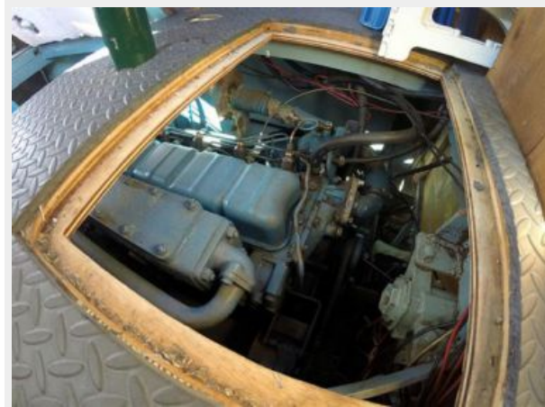
North Shore 34 Engine Room Forward
