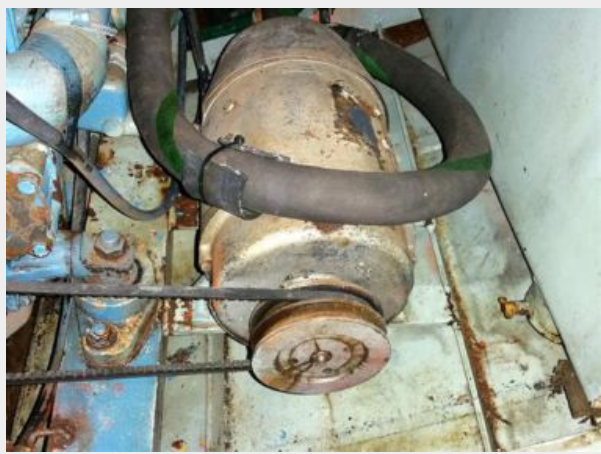
North Shore 34 Power Generator
