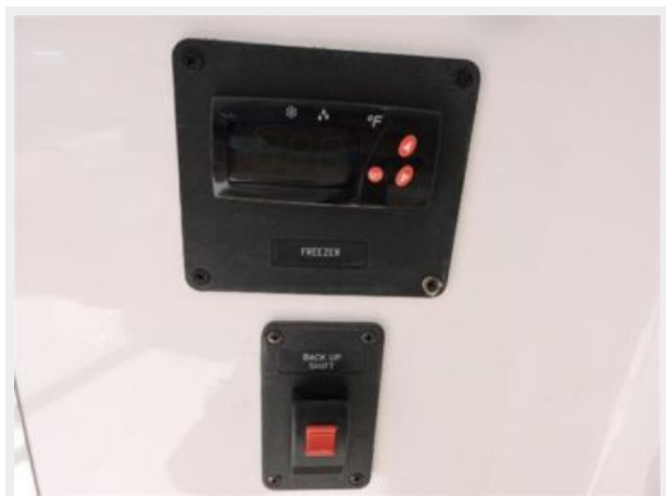
Bridge Freezer Control and Backup Electronic Controls Switch
