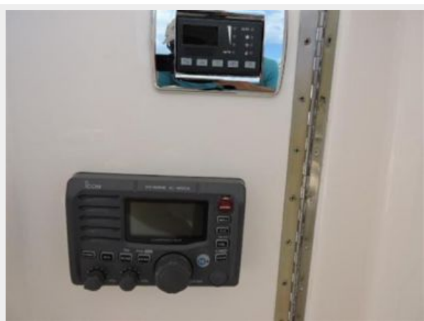
Bridge Air Conditioning Control and Icom M-504 VHF Radio
