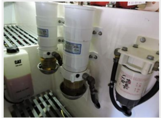
Engine and Generator RACOR Filters
