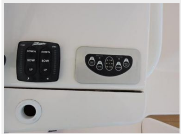
Trim Tabs and Glendening Controls Actuators
