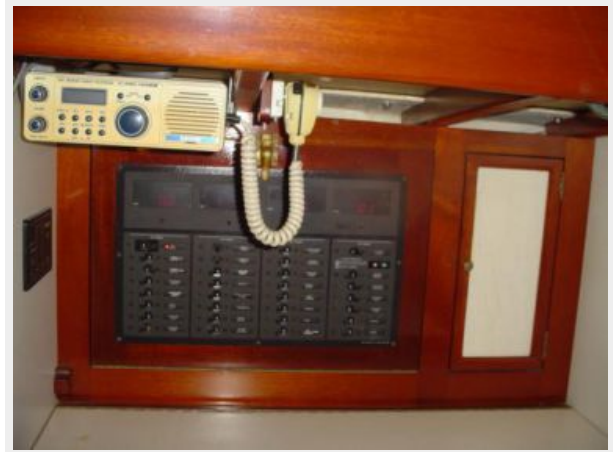
Navigation Station & Electrical Panel
