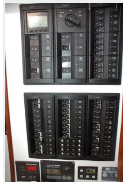
main electrical panel
