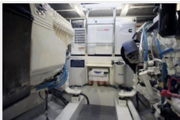
Cummins/Onan generator, oil change system
