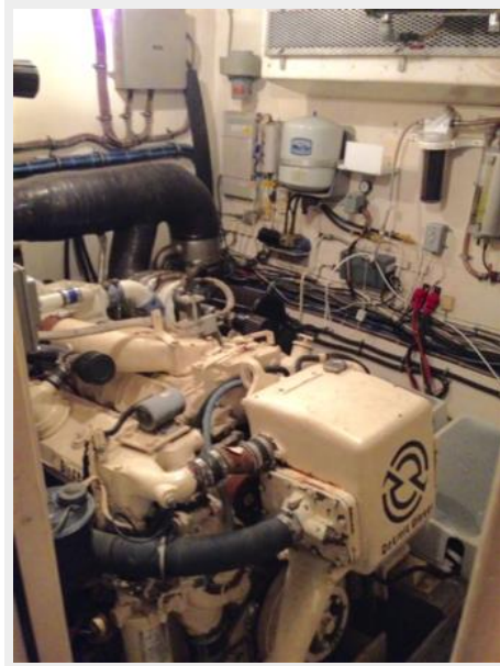
Port Engine Room
