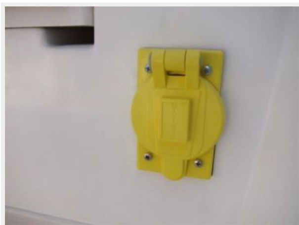
Electric Reel Outlet
