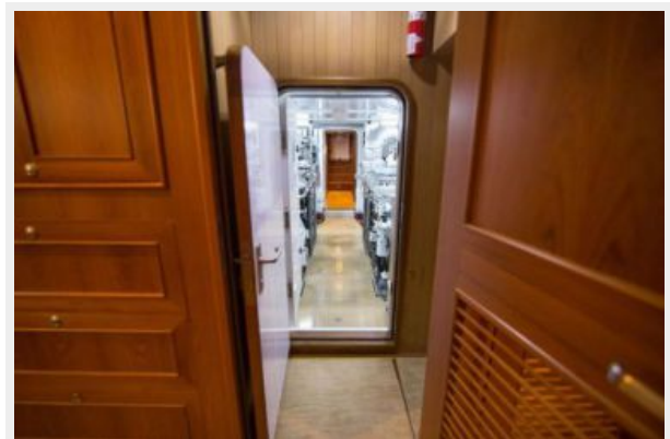
Access to Engine Room from MSR
