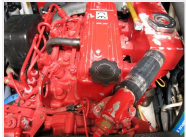
Electrical System / Equipment - Generator
