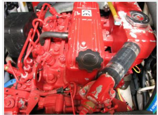
Electrical System / Equipment - Generator
