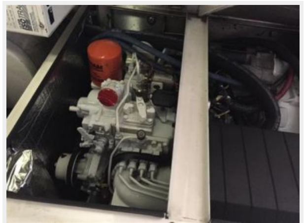
Port Generator II
