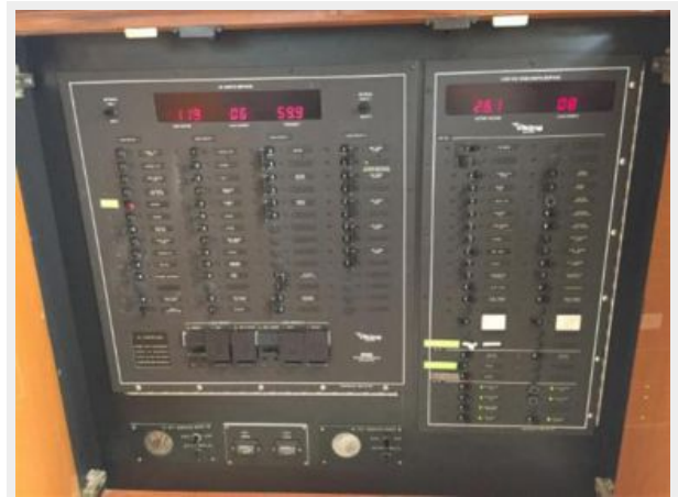
Main Electrical Panel
