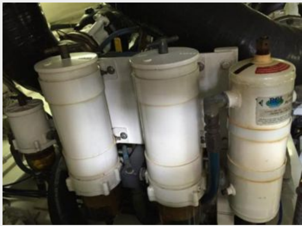
Port Engine Dual Racor Filters w/Fuel Purifier
