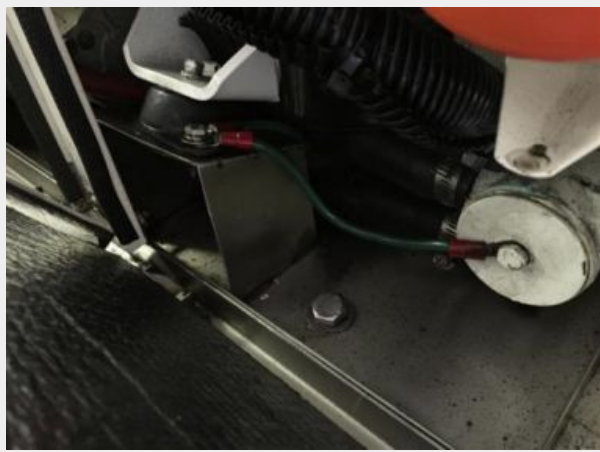
Stbd Generator II
