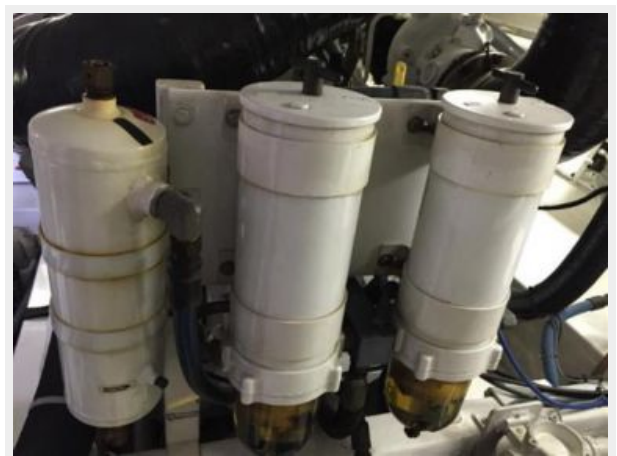
Stbd Engine Dual Racor Filters with Fuel Purifier
