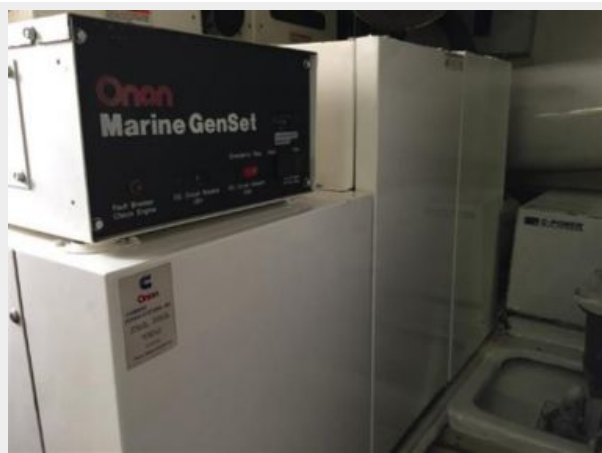
Port Generator w/Sound Shield
