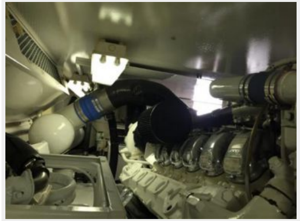
Stbd Engine Outboard Side
