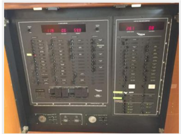
Main Electrical Panel
