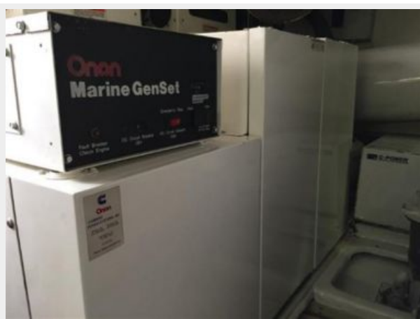
Port Generator w/Sound Shield
