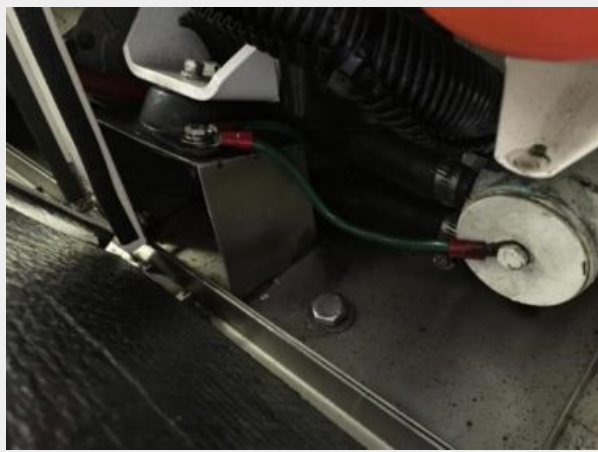
Stbd Generator II
