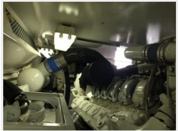
Stbd Engine Outboard Side
