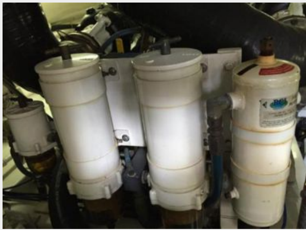
Port Engine Dual Racor Filters w/Fuel Purifier
