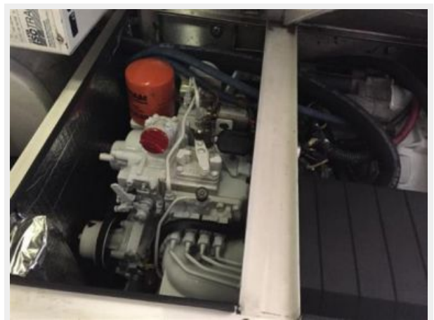
Port Generator II
