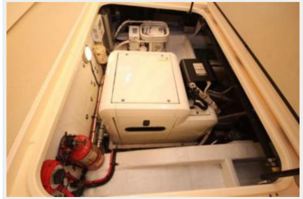
Generator Sound Box
