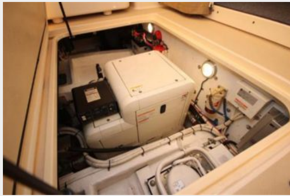
Generator w/187 hours
