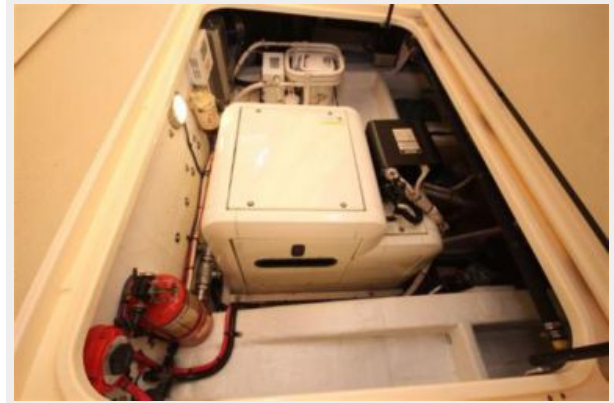
Generator Sound Box
