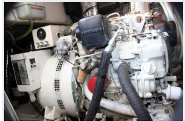
Electrical System / Equipment - Generator
