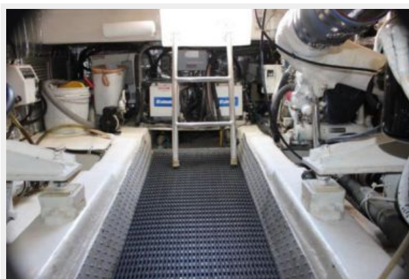
Engine & Mechanical Equipment 5 - Engine Room
