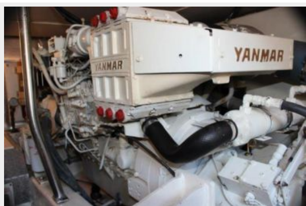
Engine & Mechanical Equipment 4 - Starboard Engine
