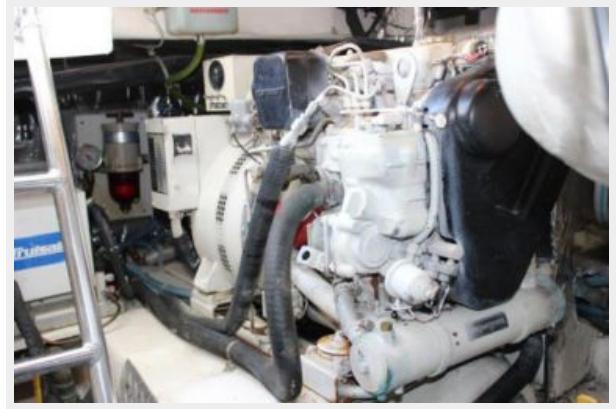
Engine & Mechanical Equipment 7 - Engine Room
