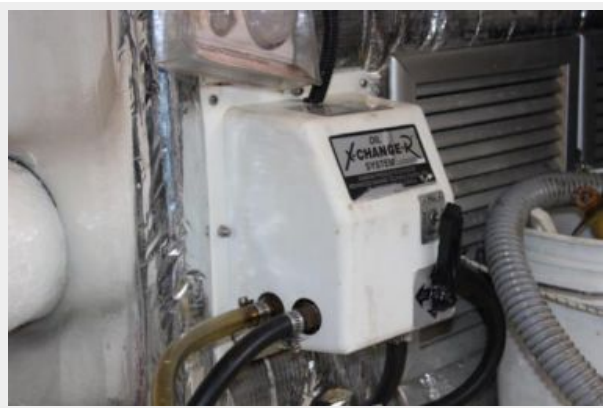
Engine & Mechanical Equipment 8 - Engine Room
