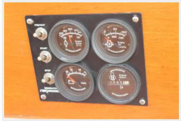
Lower Helm Generator Panel
