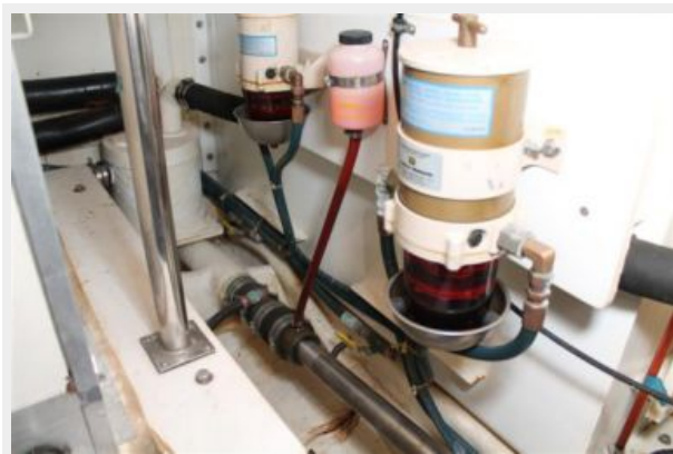
Port Shaft Seal & Fuel Filter
