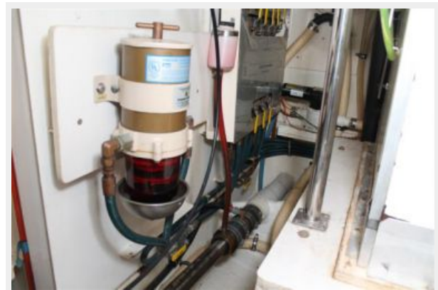
Starboard Shaft Seal & Fuel Filter
