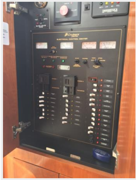
Main Distribution Panel
