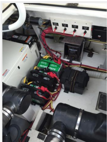
Batteries and Charger
