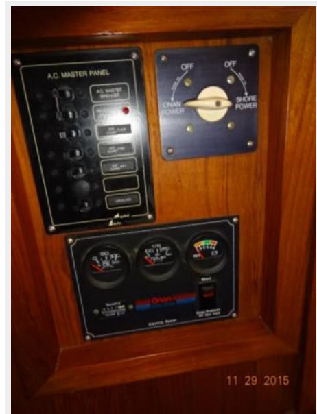
36' Monk electrical panel2
