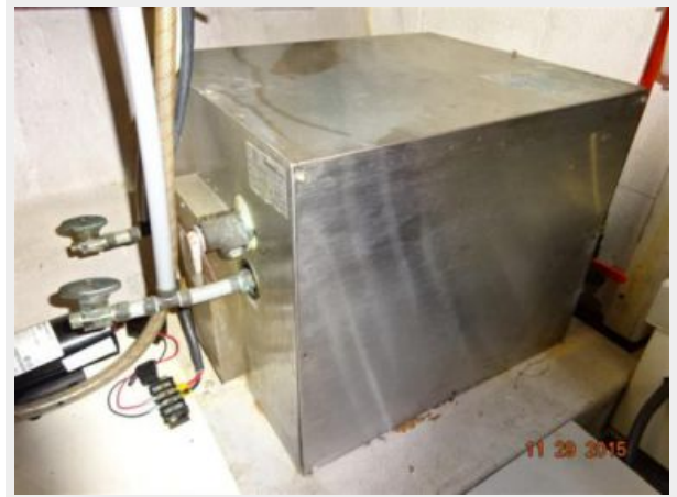
36' Monk water heater
