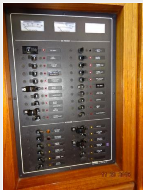
36' Monk electrical panel1
