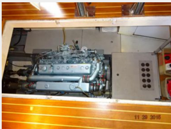
36' Monk engine room access
