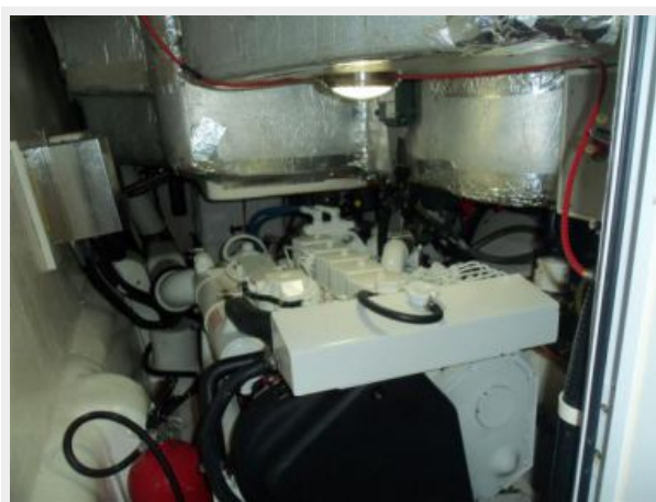
Starboard Engine Room Forward
