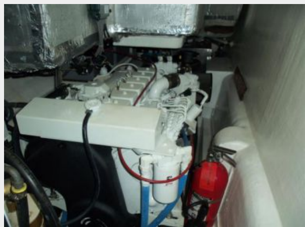
Port Engine Room Forward
