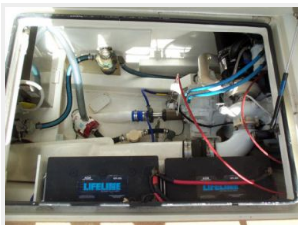
Port Engine Room Aft
