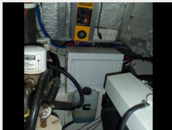
Port Engine Room
