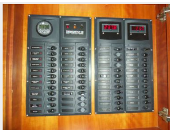
Main Electrical Panel
