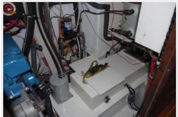
clean engine room
