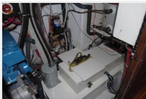
clean engine room
