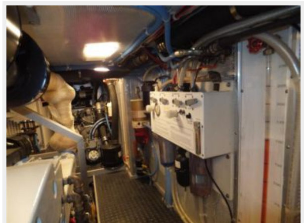
Engine room Forward
