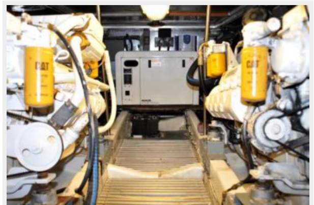
Engine Room Overview
