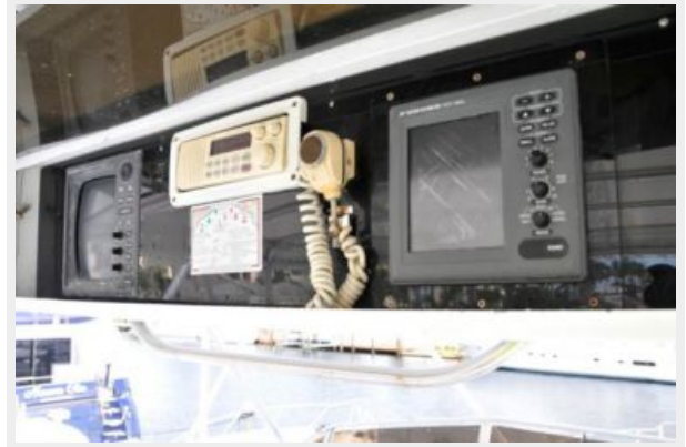
Fly Bridge Overhead Electronics 1
