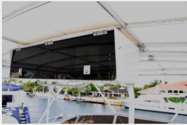
Fly Bridge Overhead Electronics Box
