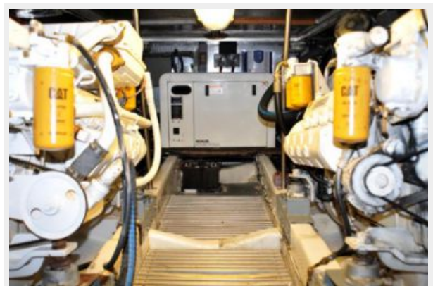
Engine Room Overview
