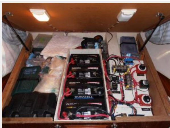
Main Bank of Batteries Under Queen Berth
