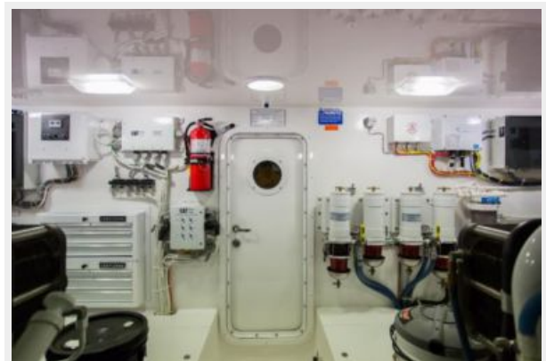
Engine Room Access to Crew Stateroom
