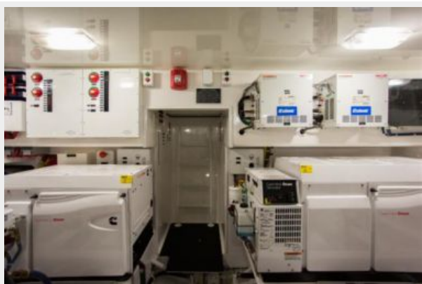
Engine Room Access to Crew Stateroom
